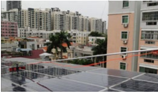
Solar panel system
